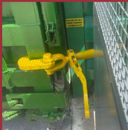
SC3000 with a modified turnbuckle.
